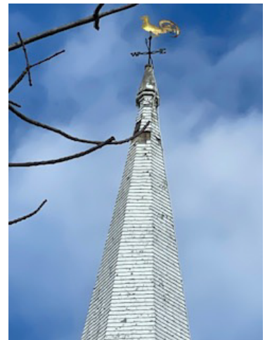
The steeple after a recent storm underscores the urgency of this priority.
